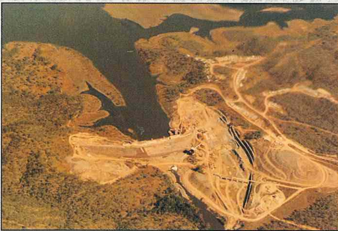
Photos of previous experiences show, Awoonga High Dam Gladstone. This was probably one of the most difficult projects grouted in Australia due to a need to accurately control uplift pressures and forces.
